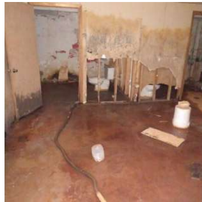
Figure 6 Building 48 basement standing water/damage
