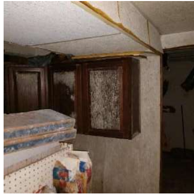
Figure 6 Mold Growth, damage
