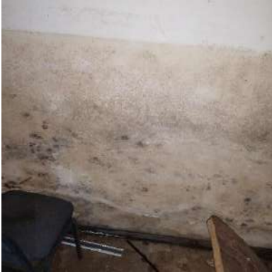
Figure 5 Mold Growth, damage
