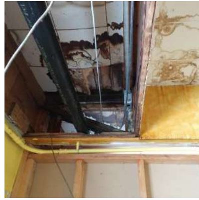
Figure 2 Building 48 roof leak
