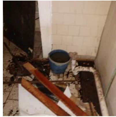
Figure 4 Building 40 Roof leak damage to Floor
