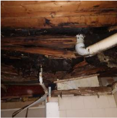
Figure 3 Building 40 Roof Leak and Roof Structure Failure
