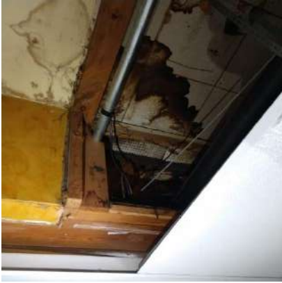
Figure 1 Building 48 Roof Leak
