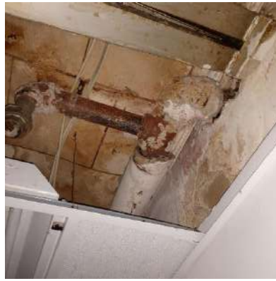
Figure 8 Possible Asbestos pipe insulation
