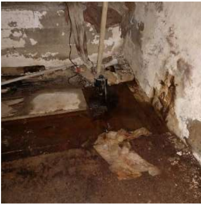
Figure 7 Failed sump, standing water
