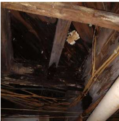
Figure 5 Building 40 Main floor damage below roof leak
