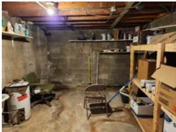
North wall of city hall, indications of water infiltration with staining on the concrete and efflorescence on the face of the cmu.
