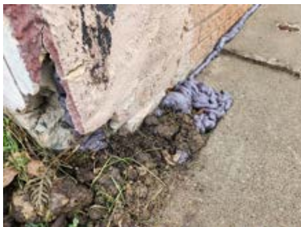
Northwest corner condition of city hall west wall and the sidewalk.
