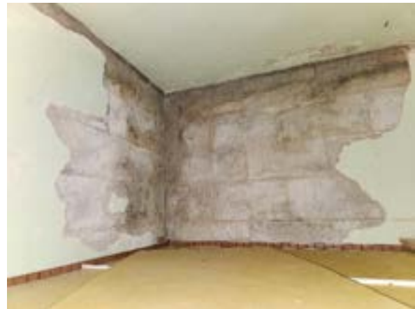
Indications of water infiltration in the bank vault on the main floor.
