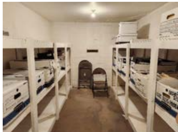
North wall of city hall, indications of water infiltration with staining on the floor and ceiling.
