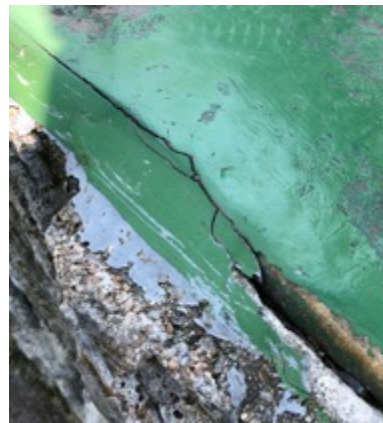
Figure 3. Detail of gray polyester resin fill material along the edge.
