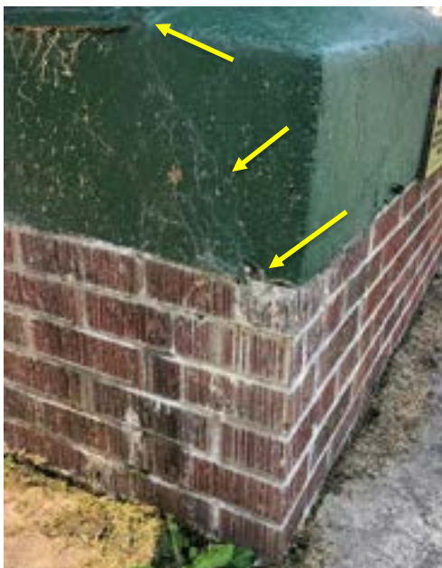
Figure 8. Proper right back corner. Yellow arrows point to spalling crack. Also note the white efflorescence on the brick and heavy layer of organic debris on the surface.
