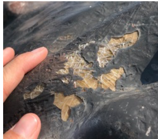
Figure 6. Detail of chips and paint loss.
