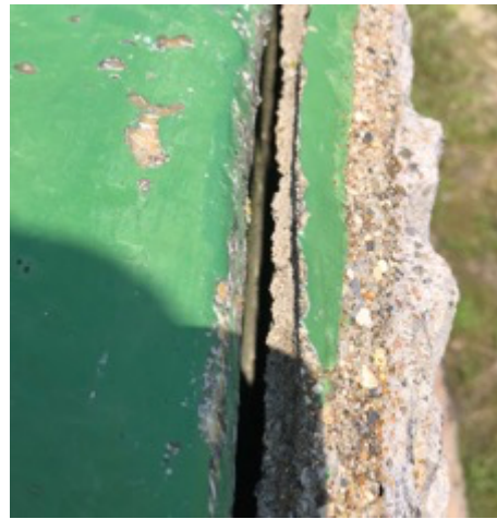
Figure 8. Detail of open gap between back stone veneer panel and concrete base.
