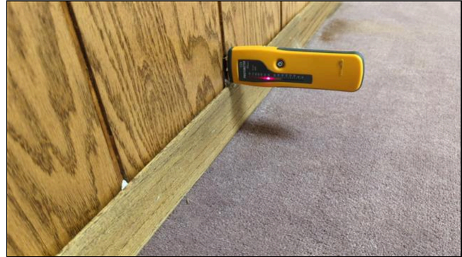
3.0 Item 6(Picture) high moisture content wall paneling
