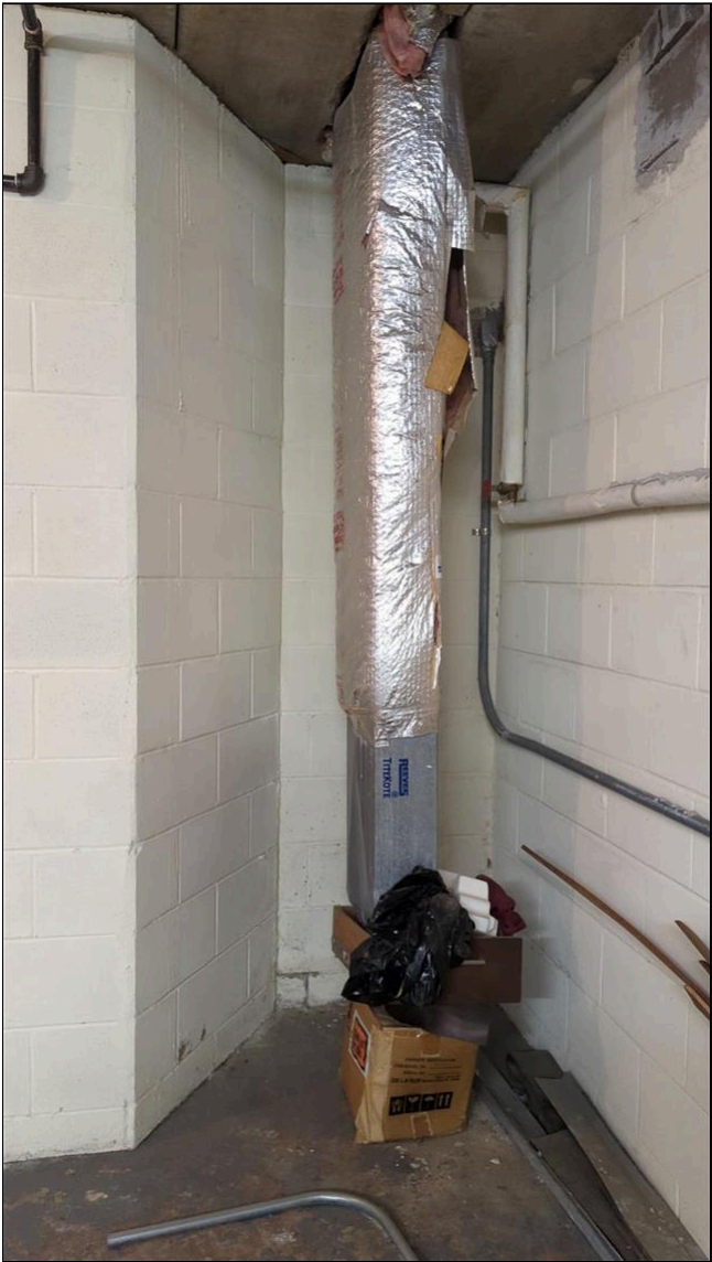
4.3 Item 4(Picture) open air return in utility room
