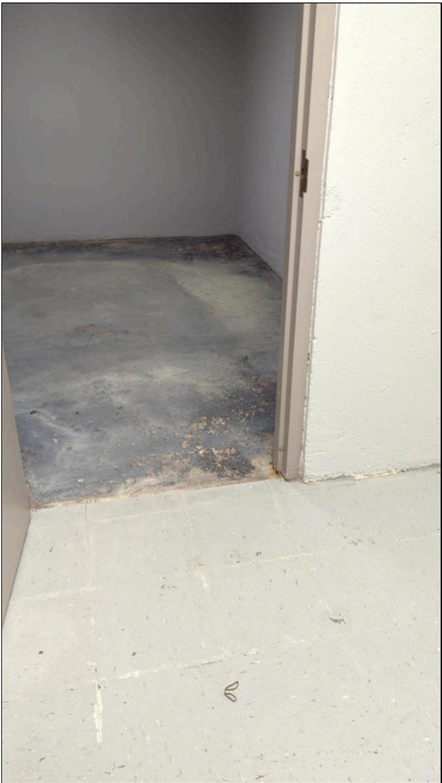
3.0 Item 2(Picture) peeling floor paint
