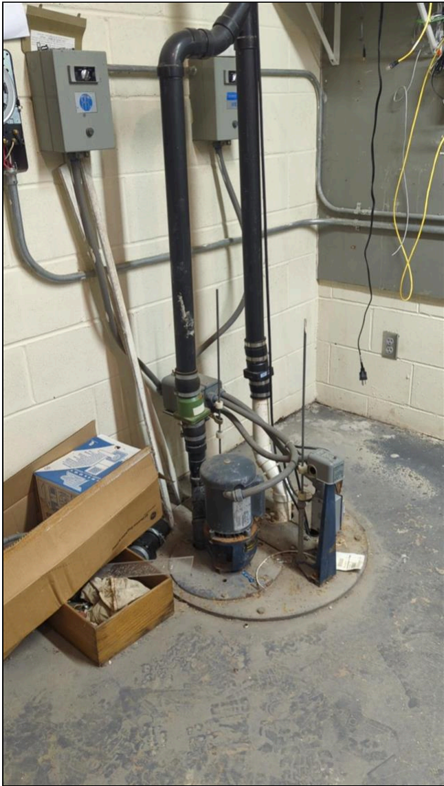
5.0 Item 2(Picture) lower level utility room lift pump
