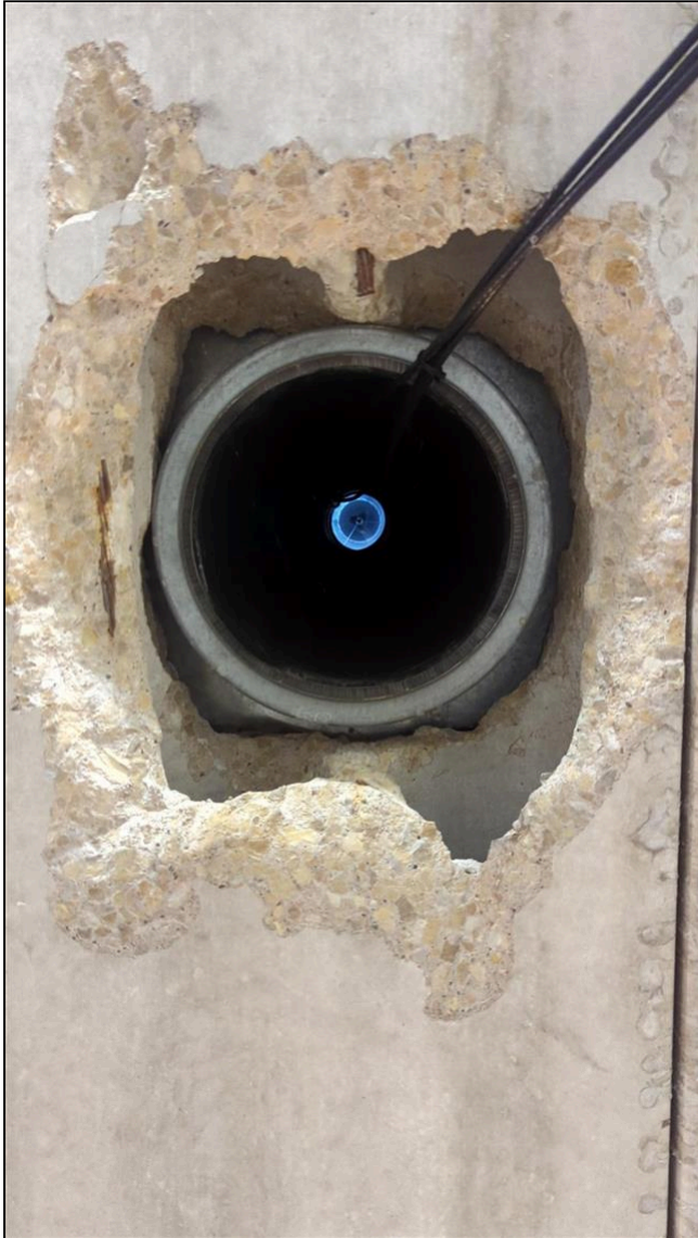
4.5 Item 1(Picture) open flue between utility room and roof
