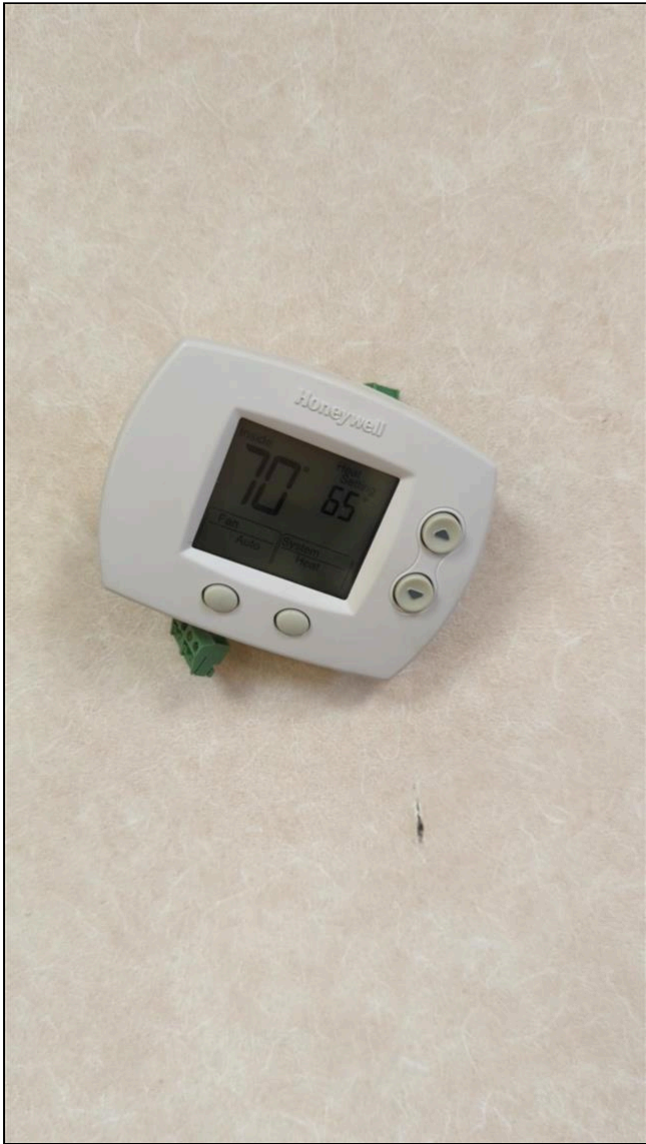
4.1 Item 1(Picture) East unit control
