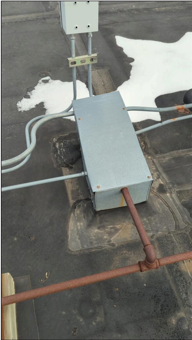
1.1 Item 7(Picture) Poorly sealed curb cover
