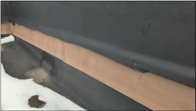
1.1 Item 6(Picture) poorly secured flashing/membrane
