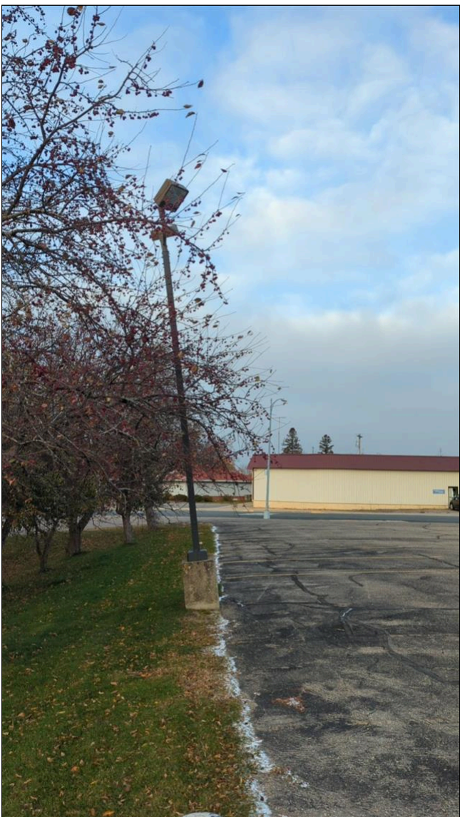
6.3 Item 2(Picture) leaning light structure
