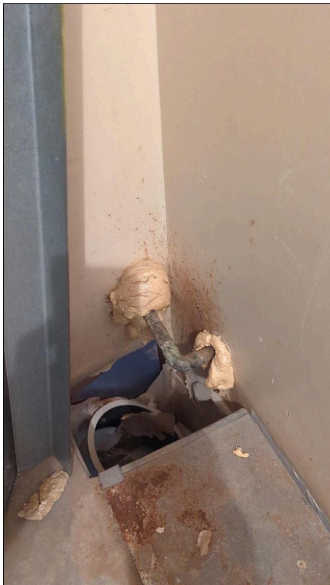
5.1 Item 3(Picture) janitor closet exterior hose bib supply
