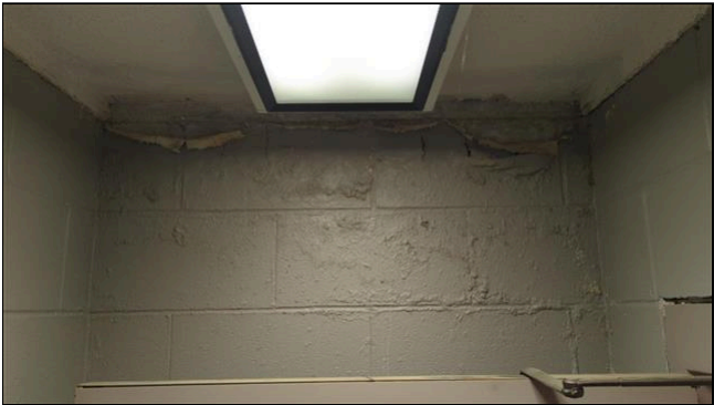
3.0 Item 10(Picture) stains/peeling wall paint
