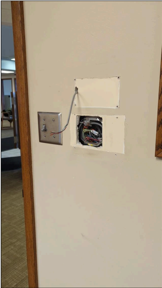
6.2 Item 3(Picture) communication wiring
