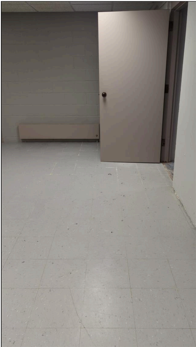
3.0 Item 1(Picture) loose floor tiling
