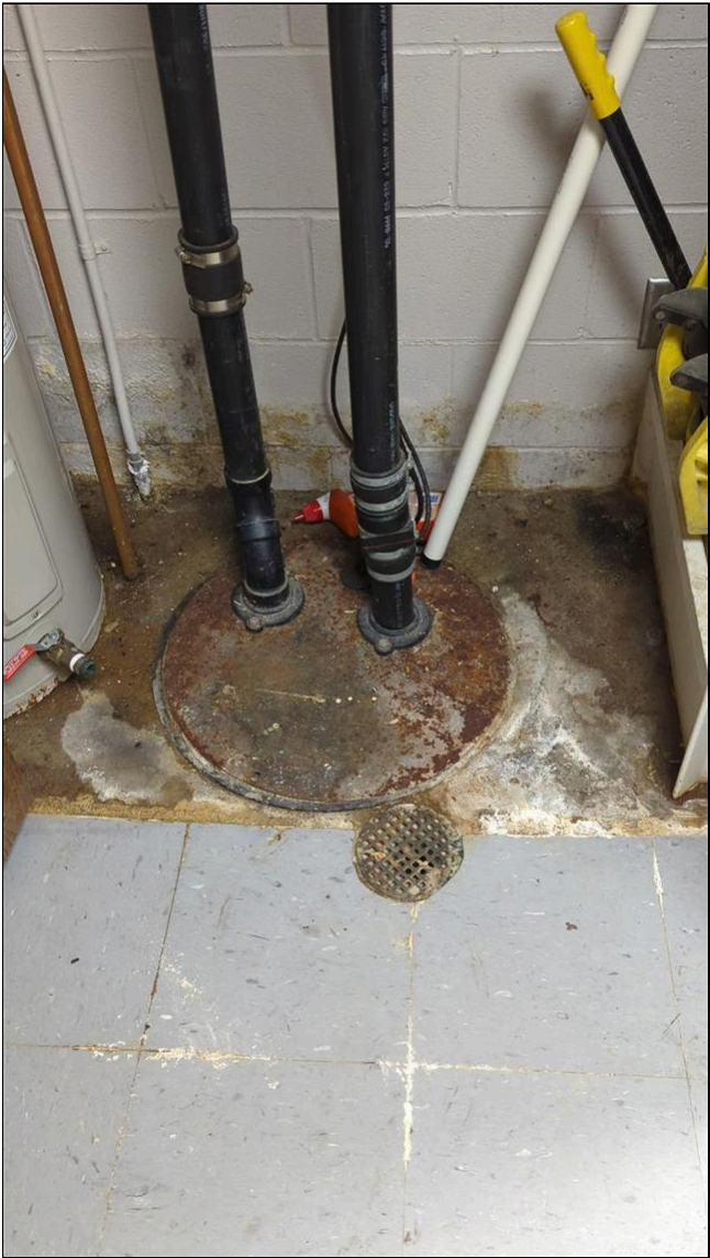
5.0 Item 3(Picture) lower level bathroom closet lift pump
