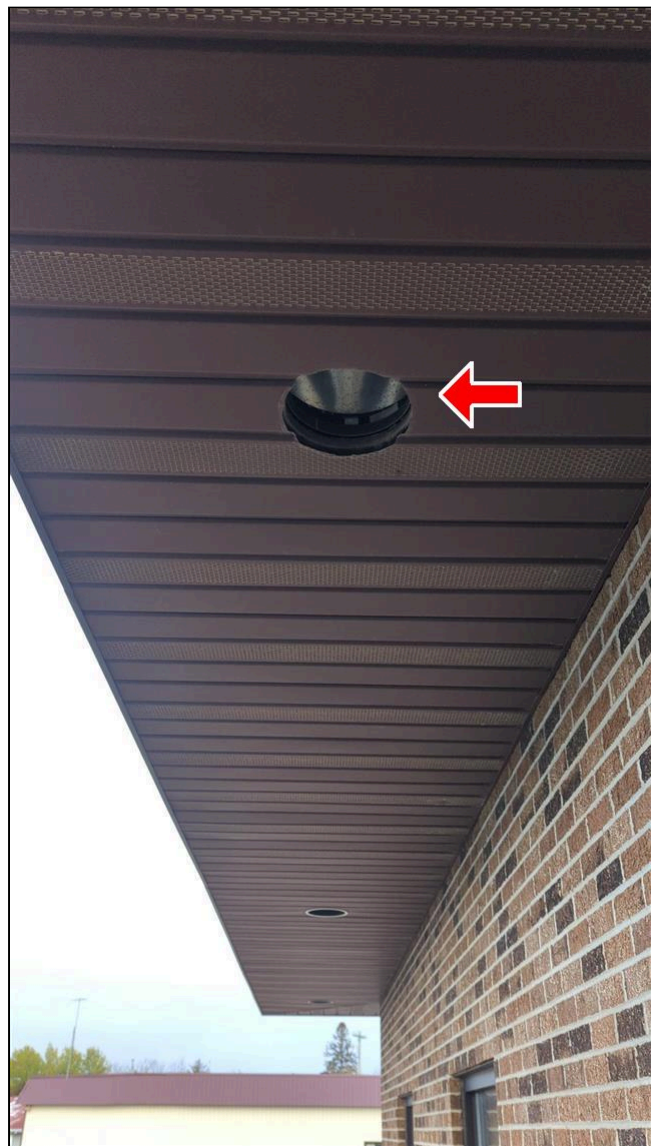
6.3 Item 1(Picture) missing light trim
