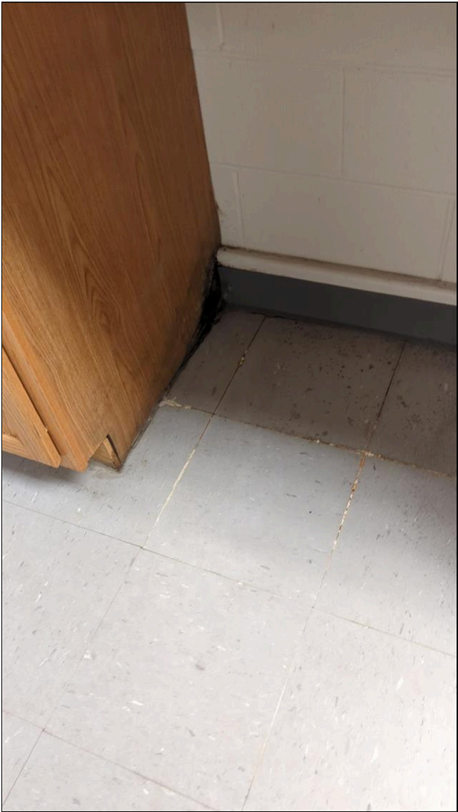
3.0 Item 8(Picture) stained cabinet base
