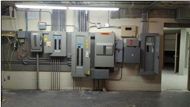
6.1 Item 6(Picture) primary electrical entrance in basement
