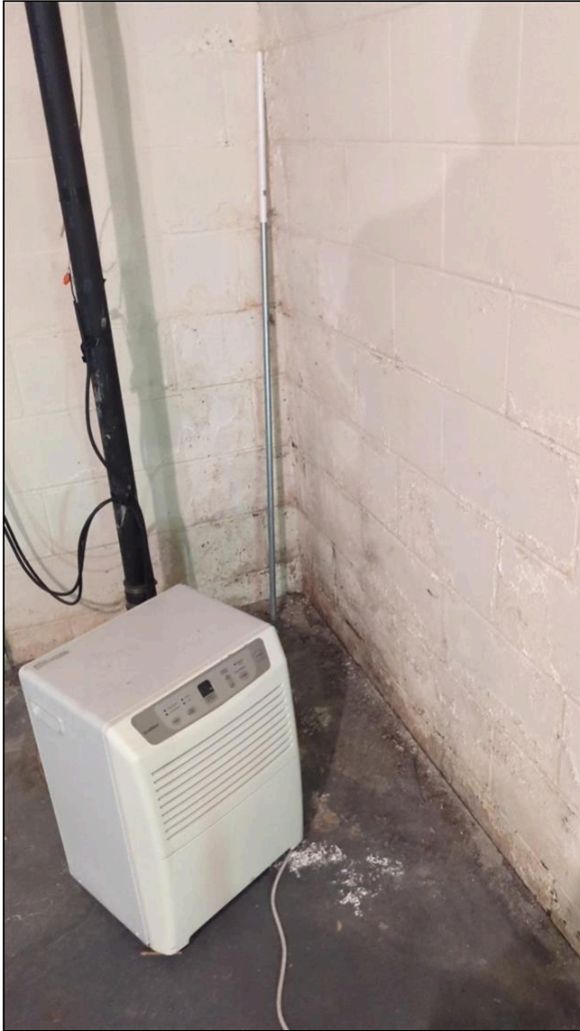
3.0 Item 5(Picture) condensation/airflow staining
