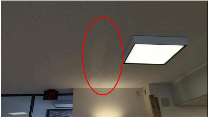
7.0 Item 3(Picture) minor repair
