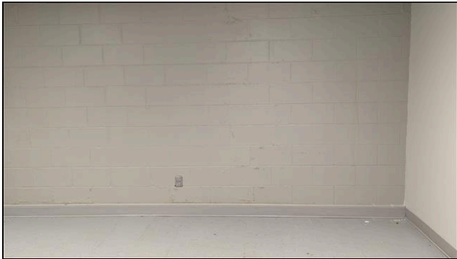
3.0 Item 7(Picture) stains and peeling wall paint
