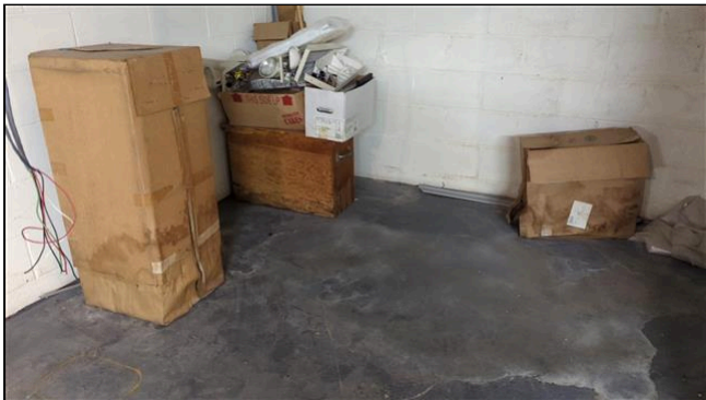
3.0 Item 3(Picture) stained floors and cardboard items
