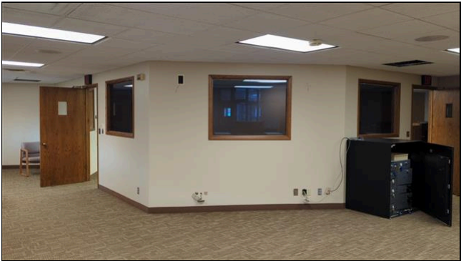
4.1 Item 2(Picture) no thermostat present in back work area?
