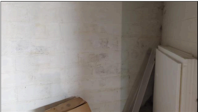
3.0 Item 4(Picture) wall stains/efflorescence
