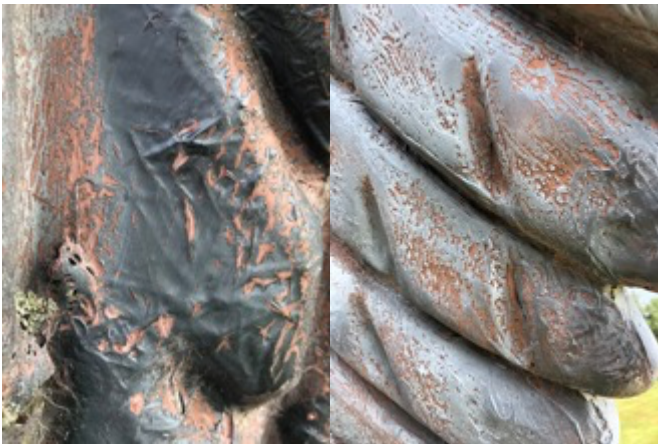
Figure 5. Examples of drying cracks/ alligatoring.
