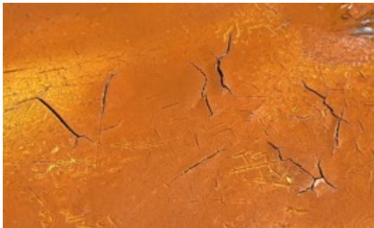
Figure 2. Detail of small cracks that extend through the paint layers and the fiberglass resin. Cracks are less than 1 inch. Also note some original yellow paint visible through the orange overpaint along the left side of the image.
