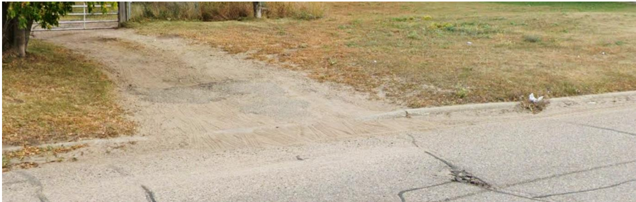
Figure 14: Sediment loading onto A Street from driveway in Red Lake.
