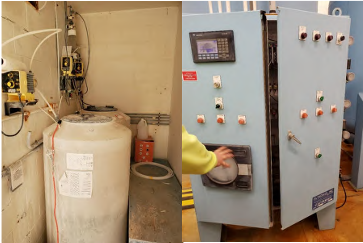
Figure 2-4 Water Treatment Facility Equipment
