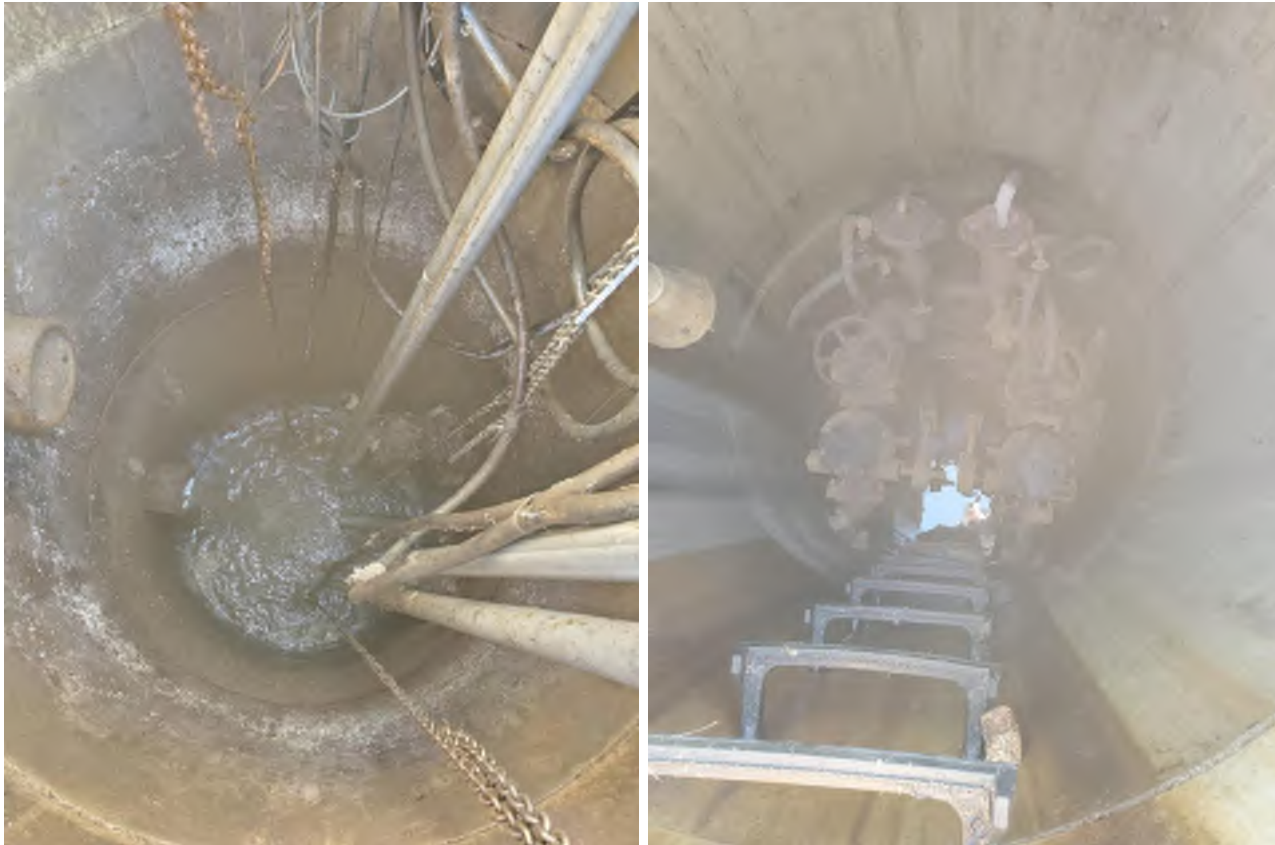
Figure 2-7 Main Lift Station (lift station 1)
