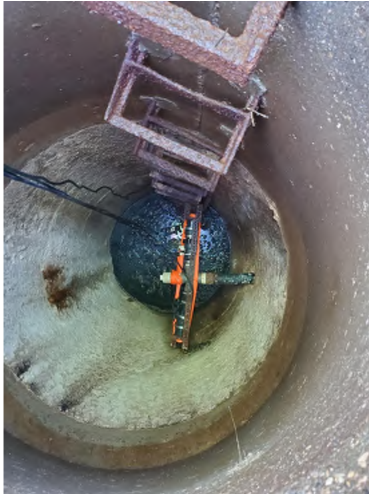
Figure 2-8 Drake Motel Lift Station (lift station 3)
