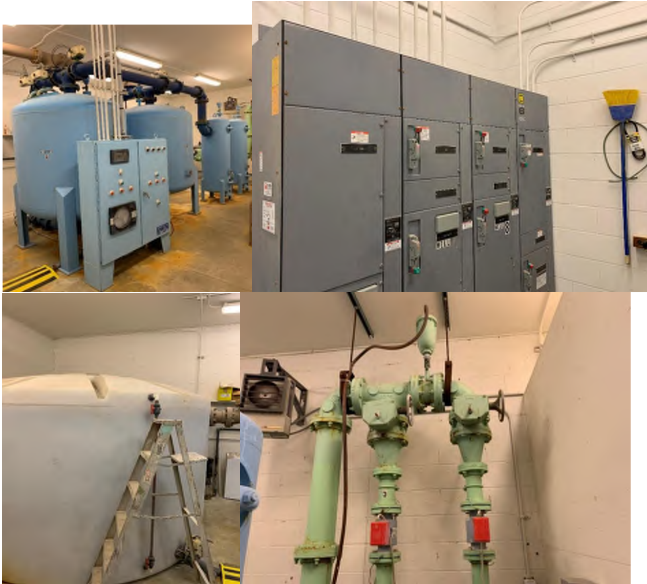
Figure 2-5 Water Treatment Facility Equipment
